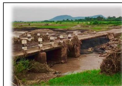
Heavy rain at the start of the year caused flooding. Here the bridge at Mkoka has been swept away in the powerful flow. Fields and young plants were also left covered in mud. Please pray for a good harvest despite these floods, and for food for all this year.
